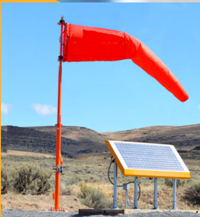
Remote power and sign lighting
